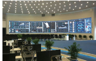
Network Operation Centres (NOC)
